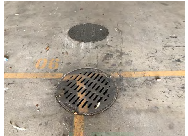
12. View of floor drains leading to the clarifier in the enclosed area (Photo 11).
