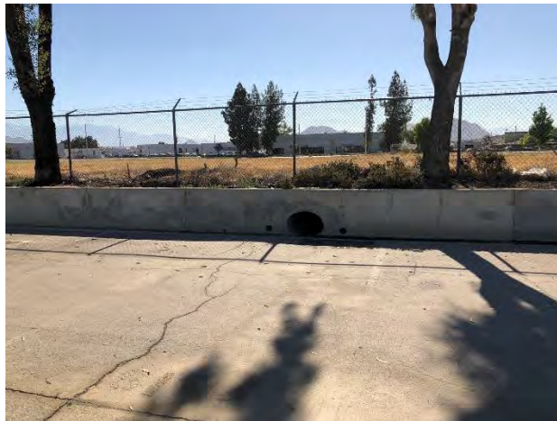
5. View of the stormwater runoff culvert at the northeastern edge of the Site facing east.
