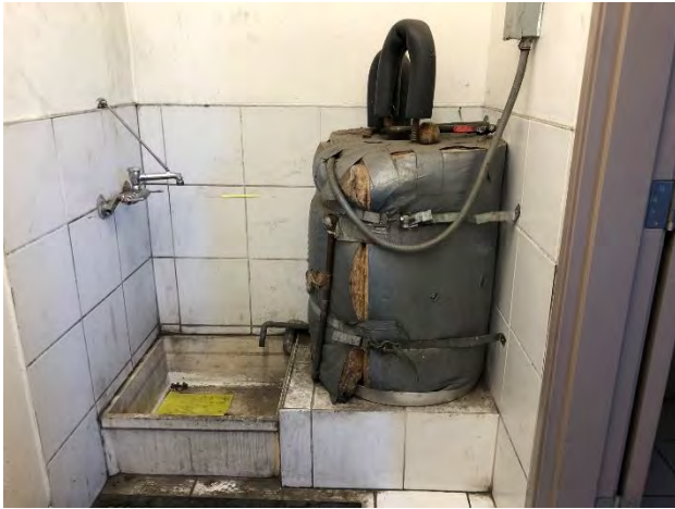
49. View of the maintenance closet and mop sink within the 200 Sinclair Street building.
