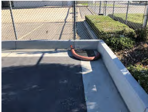
35. View of a catch basin northeast of 200 Sinclair Street reportedly leading to a dry well.
