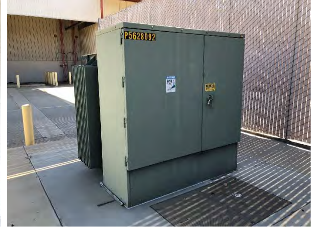
9. View of typical pad-mounted transformer south of the building.
