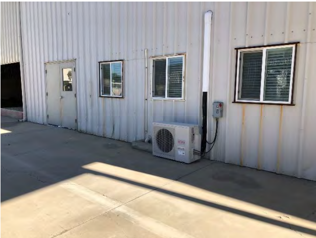
10. View of the wall mounted air conditioning unit outside of the Marvin offices.
