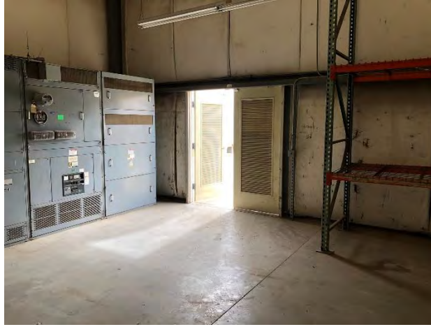
14. View of the electrical room along the south side of the 100 Sinclair Street building.
