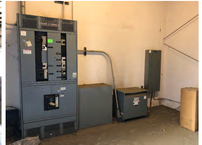
48. View of the 200 Sinclair Street building electrical room.
