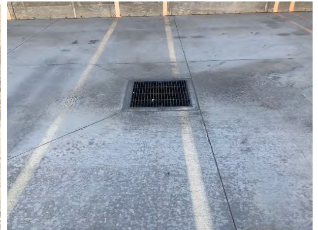
30. View of typical stormwater catch basin in the loading docks area.
