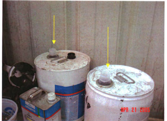
Open top containers of flammable liquid
