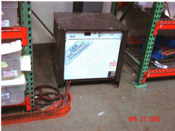
Forklift battery recharger
