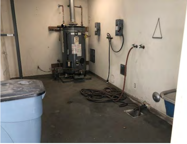
13. View of the maintenance room with floor drain in the 100 Sinclair Street building.
