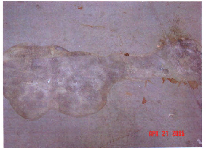
Spillage from forklift batteries
