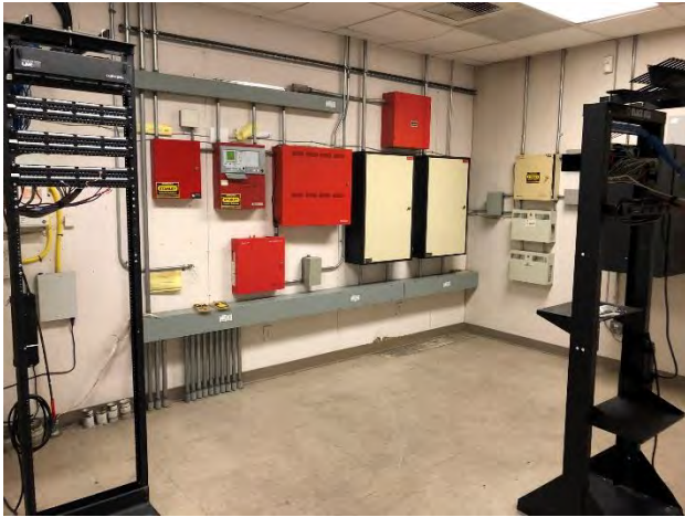
19. View of the electrical/server room in the eastern side of the 100 Sinclair Street building.
