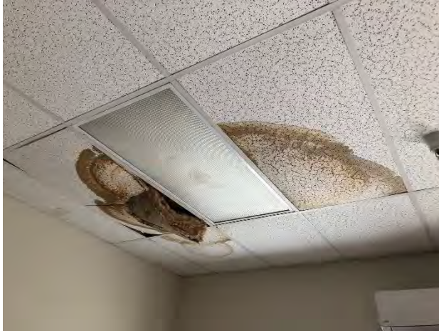
26. View of apparent ceiling water damage in the Marvin office area.
