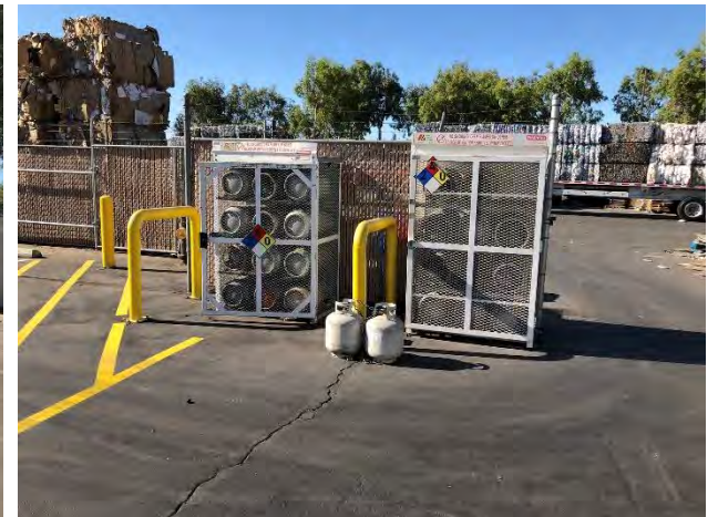
42. View of the propane storage area south of the 200 Sinclair Street building.
