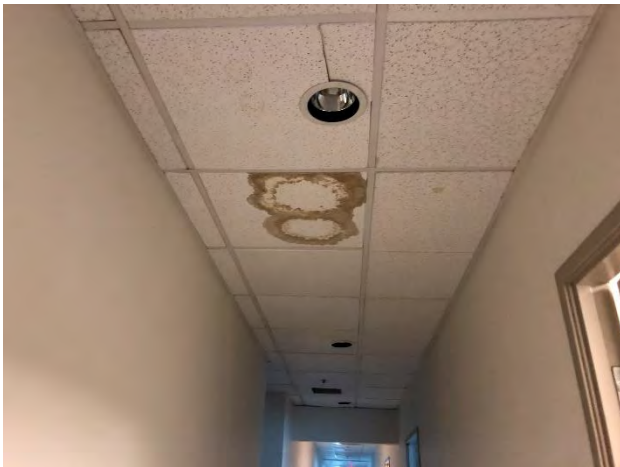
22. View of apparent water damage to the ceiling in the mezzanine office corridor.
