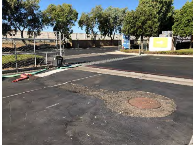
44. View of the surface completion of stormwater capture features south of 200 Sinclair Street.
