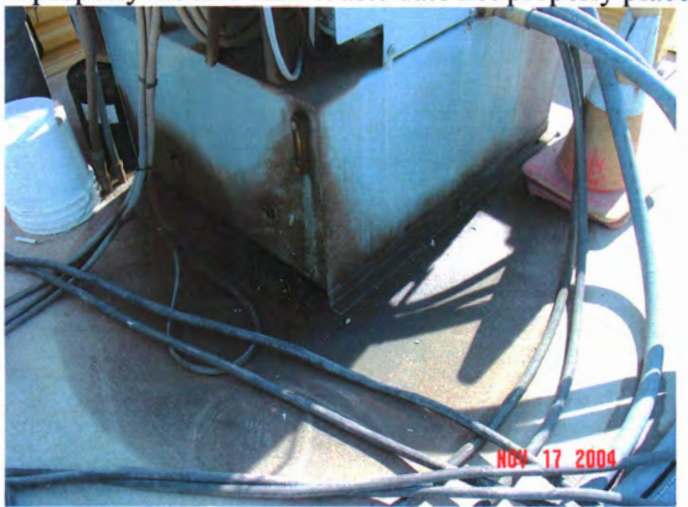
Spillage of oil onto concrete pad
