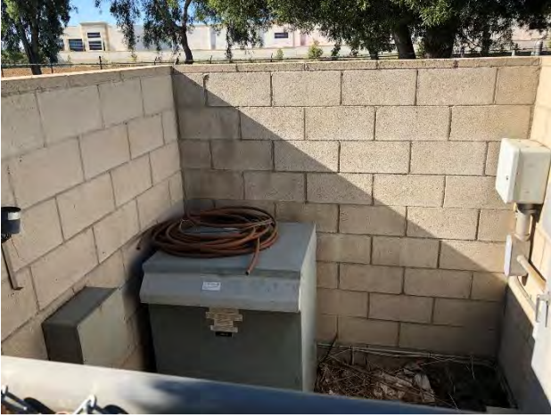
43. View of the transformer area south of the 200 Sinclair Street building.
