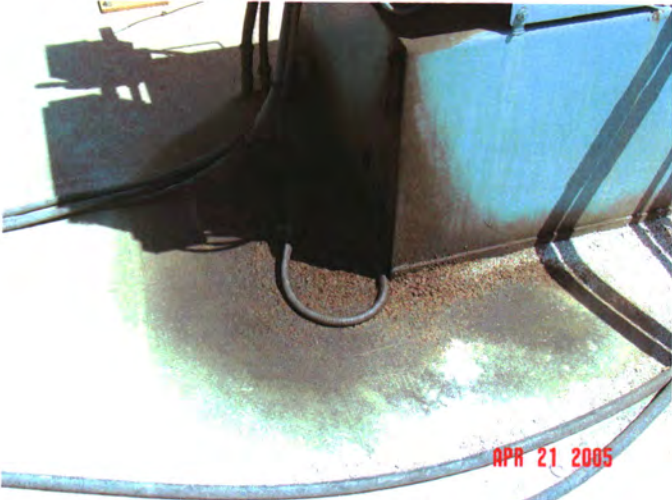
Spill identified last inspection
