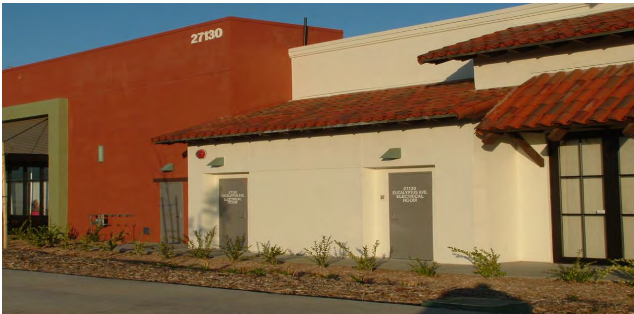
Built in Utility Equipment Room
