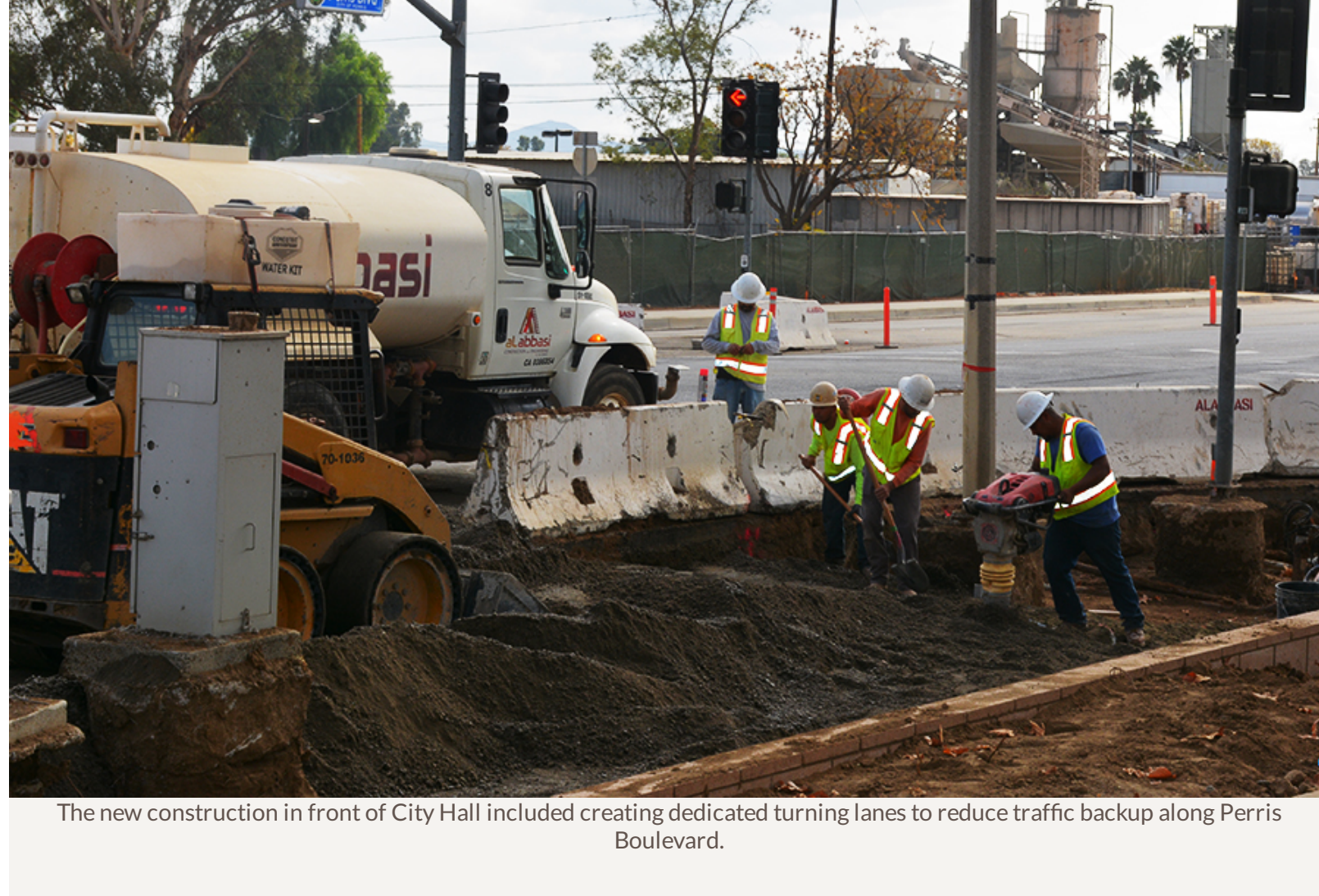
The new construction in front of City Hall included creating dedicated turning lanes to reduce traffic backup along Perris Boulevard.
