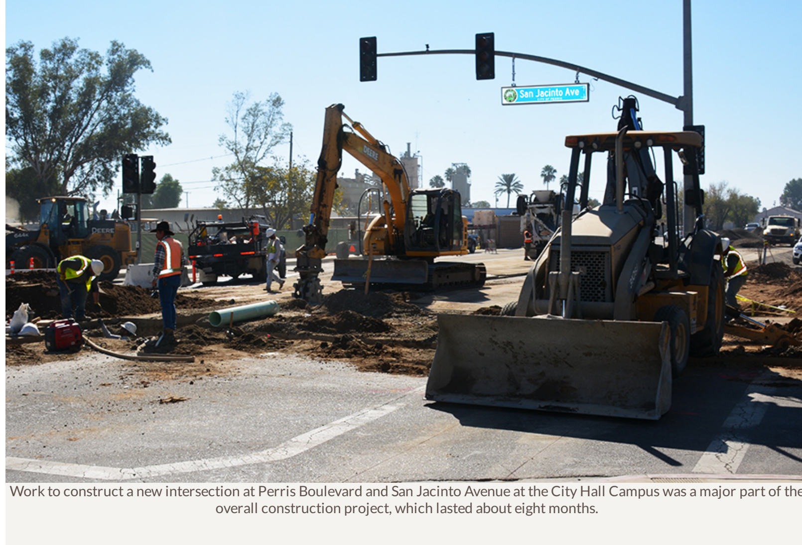
Work to construct a new intersection at Perris Boulevard and San Jacinto Avenue at the City Hall Campus was a major part of the overall construction project, which lasted about eight months.
