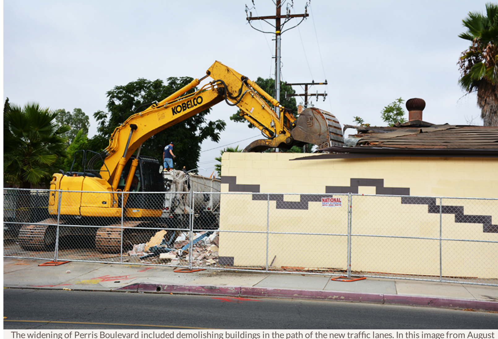
The widening of Perris Boulevard included demolishing buildings in the path of the new traffic lanes. In this image from August 2017, a bulldozer chops a structure near Perris Boulevard and Second Street.
