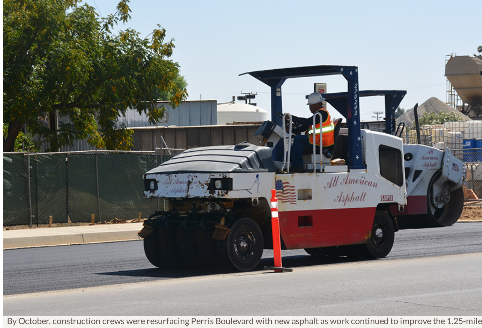
By October, construction crews were resurfacing Perris Boulevard with new asphalt as work continued to improve the 1.25-mile of roadway through Downtown.
