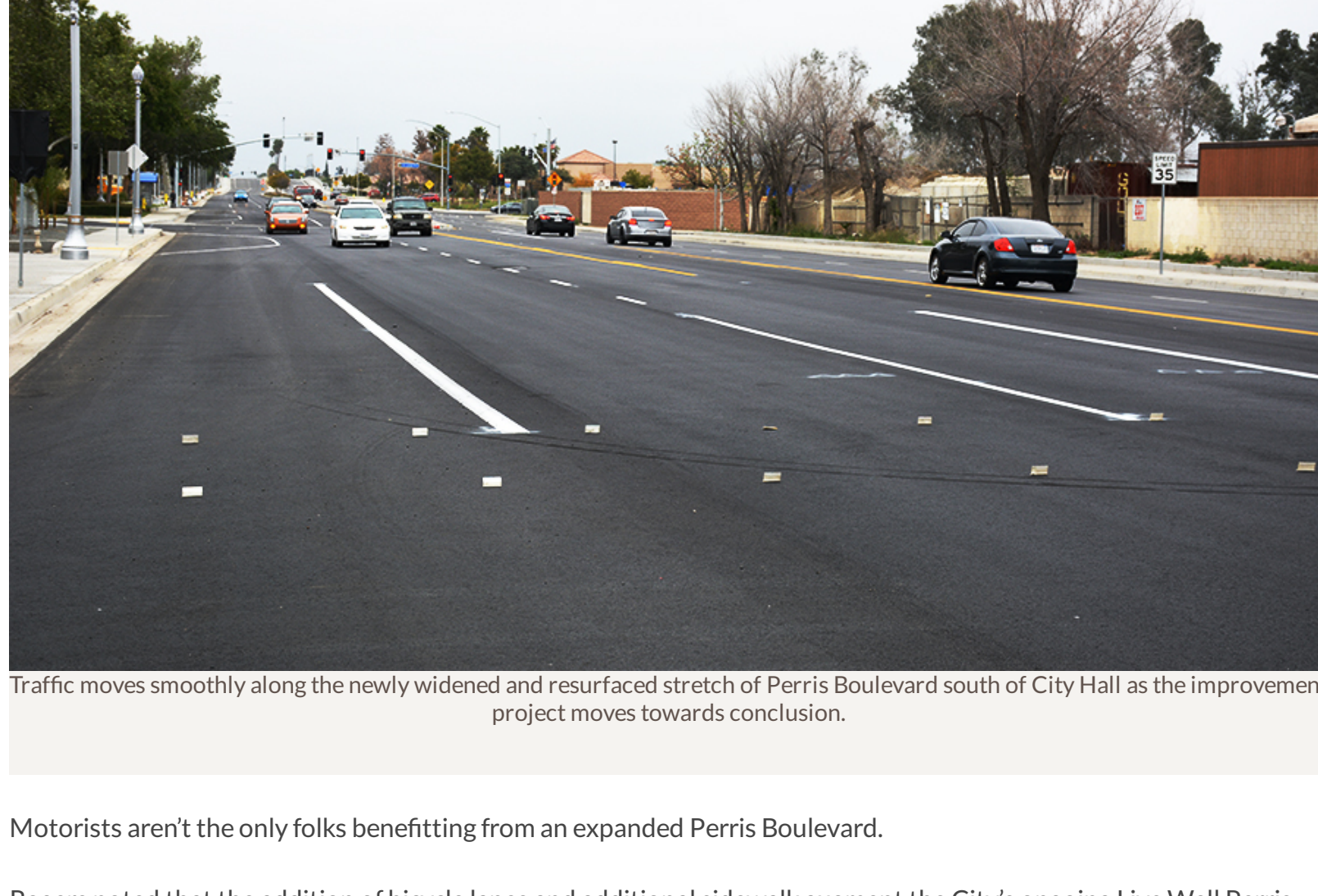
Traffic moves smoothly along the newly widened and resurfaced stretch of Perris Boulevard south of City Hall as the improvement project moves towards conclusion.
