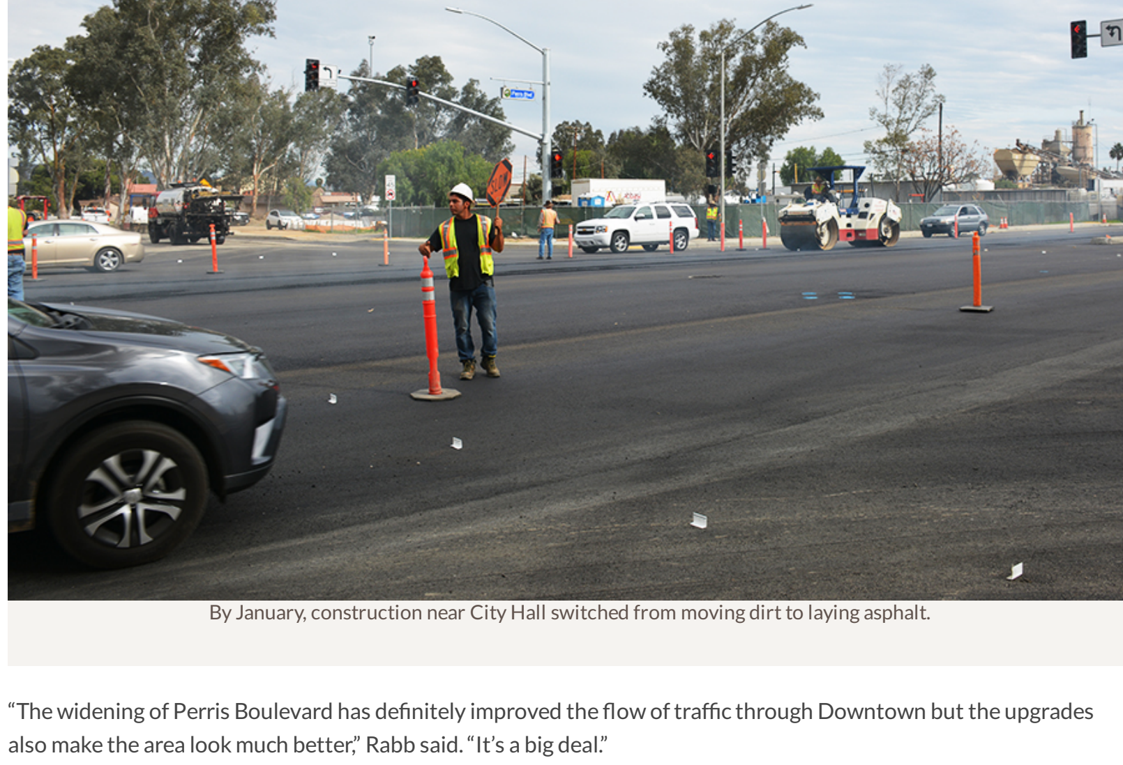
By January, construction near City Hall switched from moving dirt to laying asphalt.
