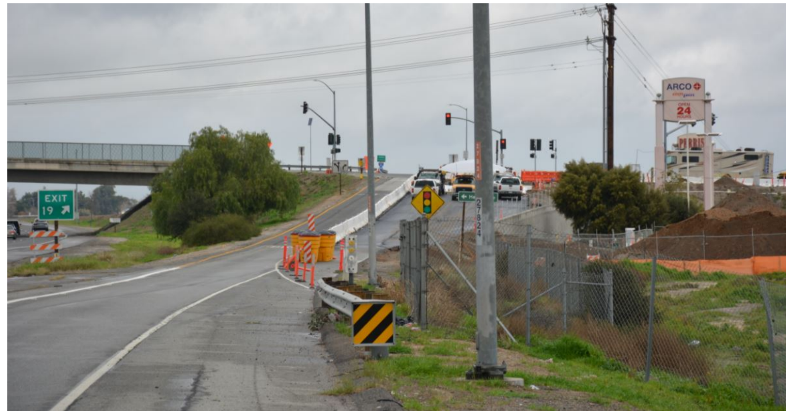
Improvements to the Interstate 215 interchange at Nuevo Road are expected to be completed by early April 2017.
