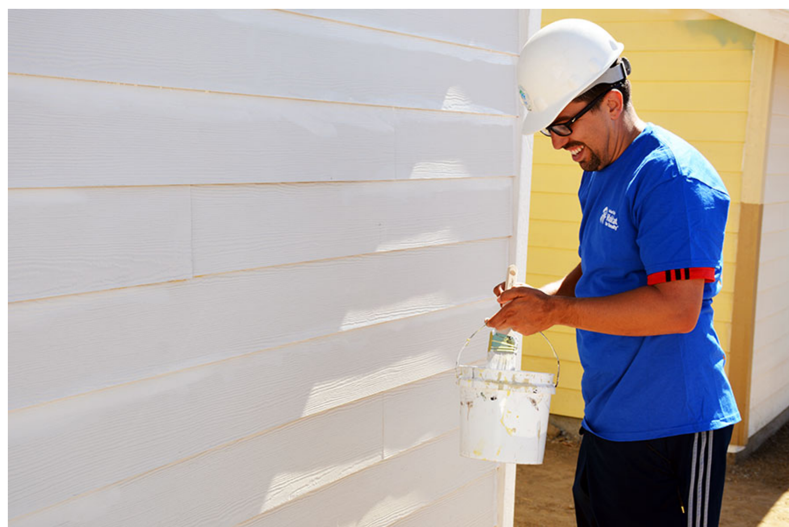
Perris City Councilman Malcolm Corona slaps a coat of paint on the exterior siding of a Habitat for Humanity home on South Street in Perris.
