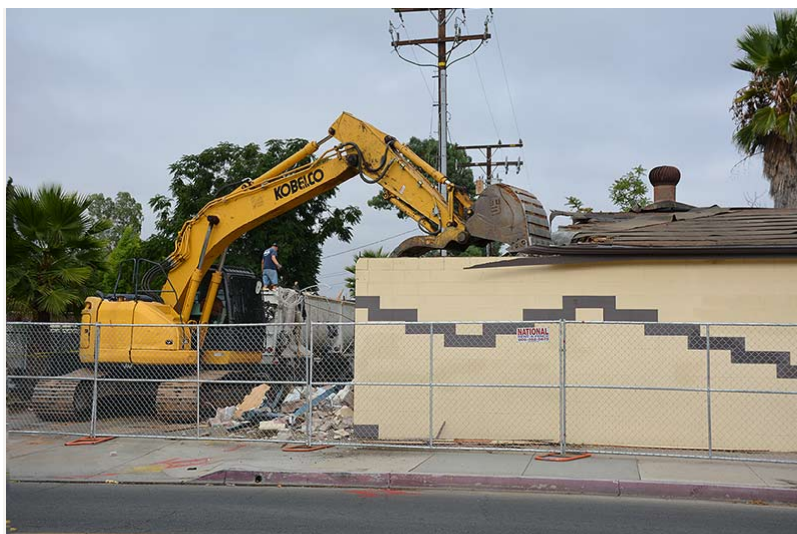
A building known as "The Boulevard" is taken down to make way for a new lane along Perris Boulevard.
