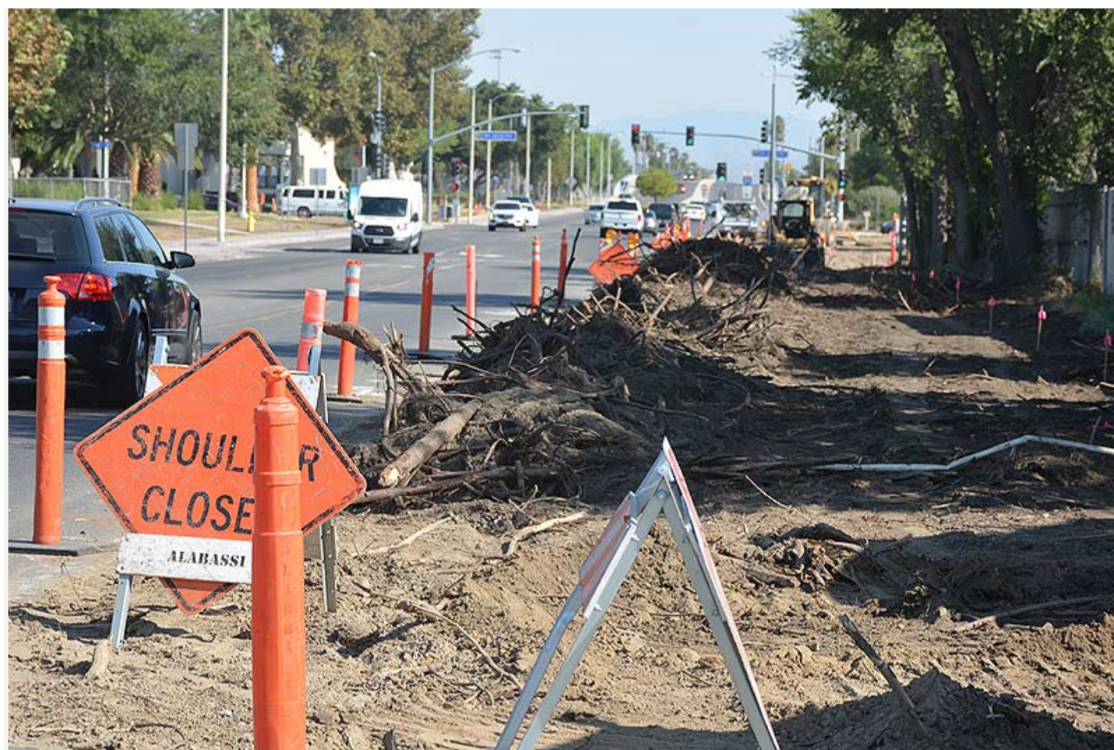
Construction work along Perris Boulevard is underway to widen the traffic arterial that cuts through Downtown Perris.
