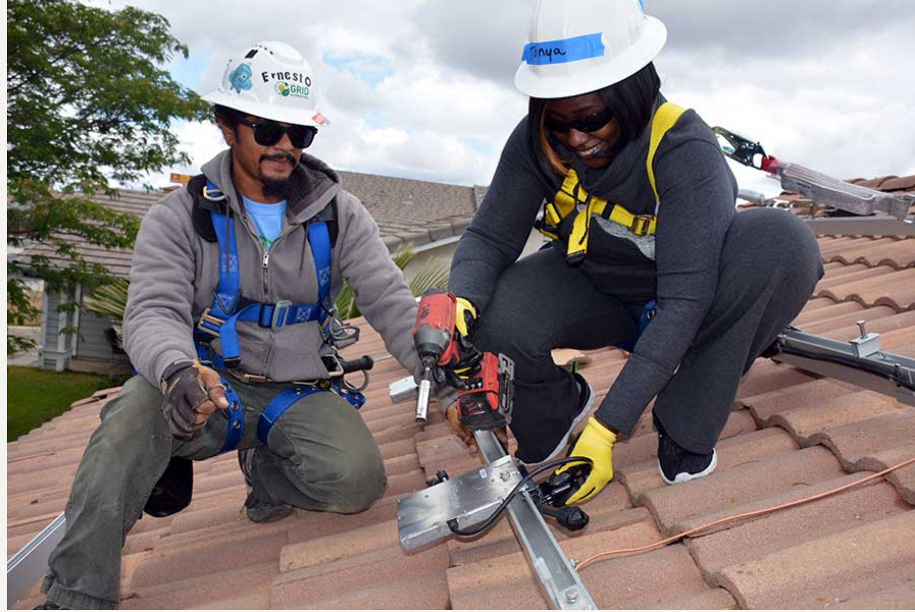
Perris City Councilwoman Tonya Burke and GRID Alternatives supervisor Ernesto Rochester install a solar panel May 7 at the residence of Monica Cruz, who expects to save thousands of dollars in electricity bills in the coming years.
