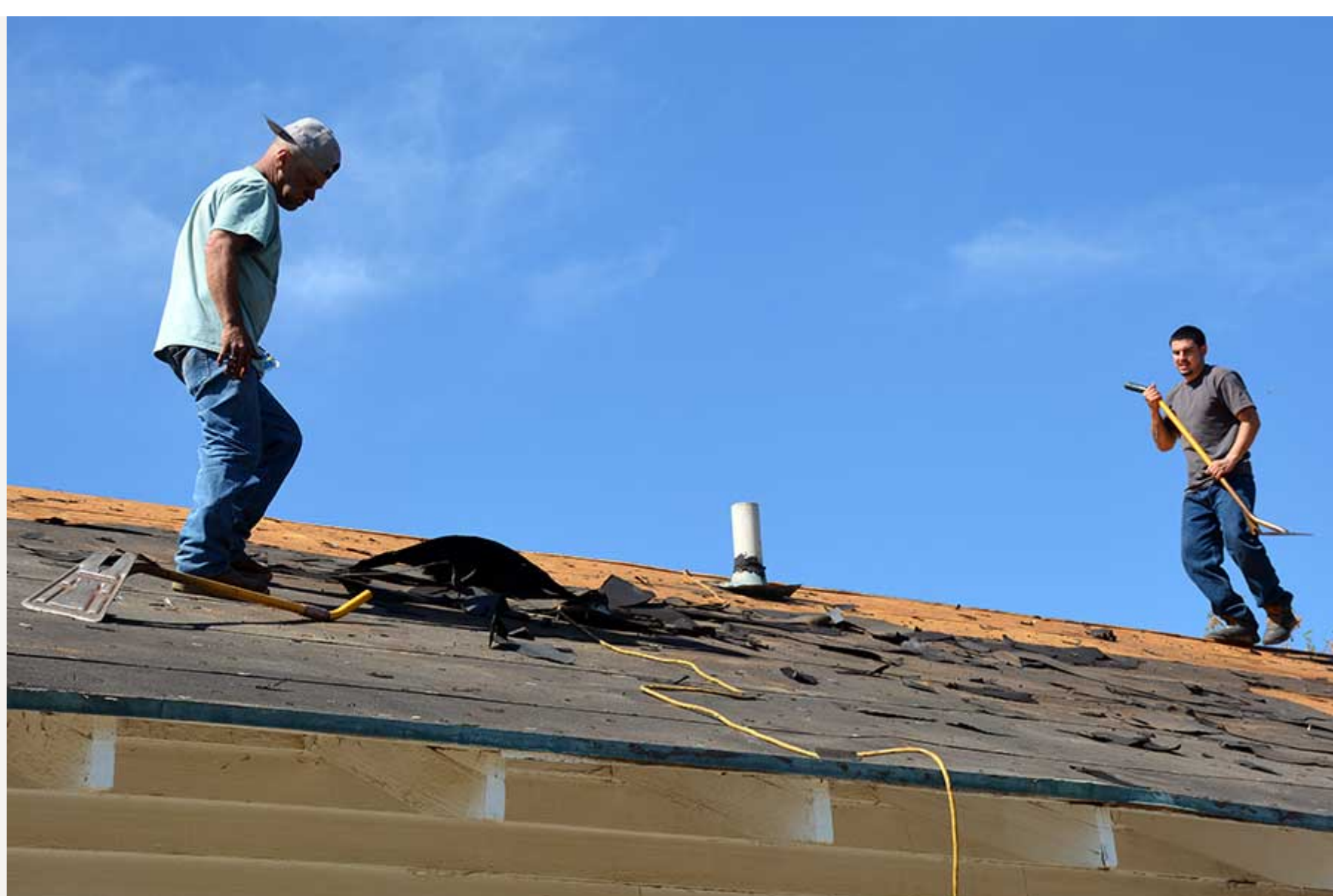
Workers remove a damaged roof prior to replacing it at the Dora Nelson African-American Art and History Museum.
