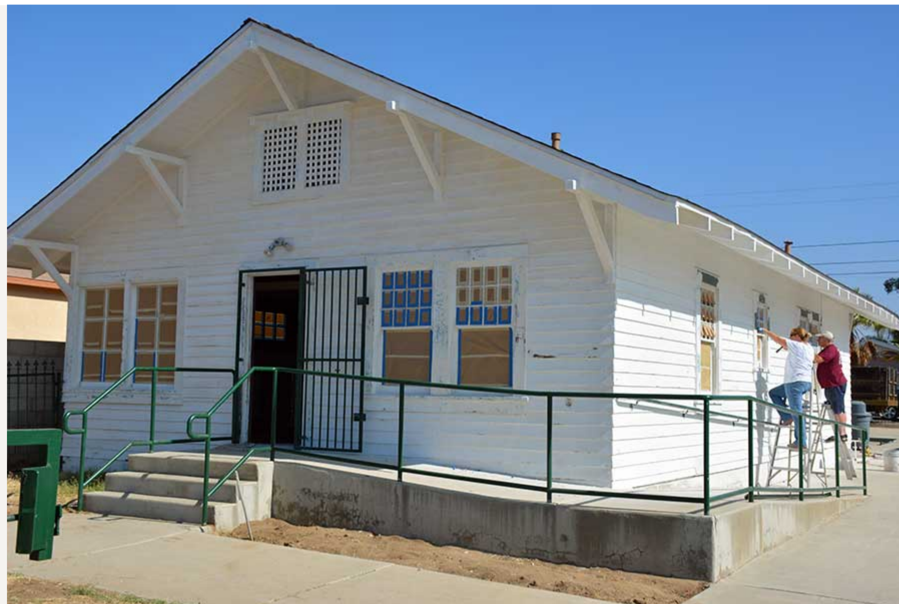
The Dora Nelson African American Art & History Museum has been upgraded with a new roof, new interior and exterior painting, new walls, flooring and plumbing. The museum will host an August 3 reception from the Association of African-American Museums.
